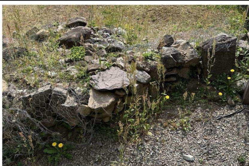
S6.I3 Late Bronze Age Wall in need of restoration near the Stelae Pit.
