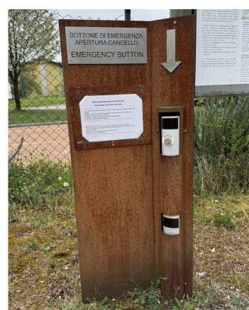
S4.15 The Emergency Release Button to open the gates in case of emergency
