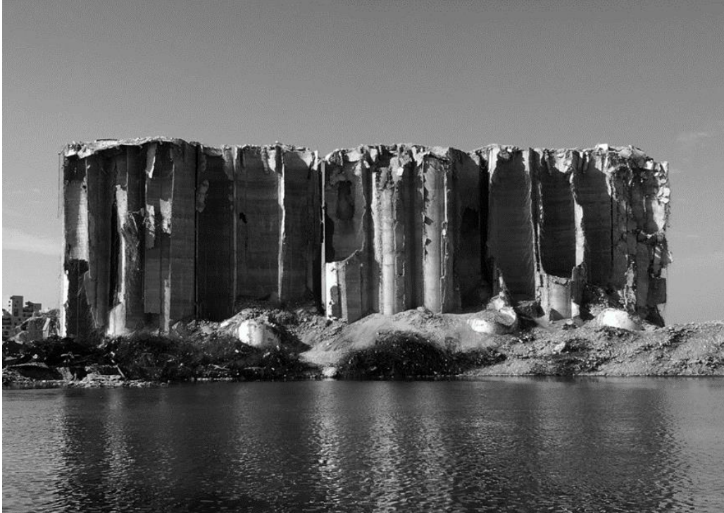
Figure 18: Shows the destruction of the grain silos in the Port of Beirut after the explosion (Photo courtesy of Emmanuel Durand, 2020).
