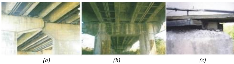
Figure 2-7 A few damage scenarios during the 1990 Chi-Chi earthquake; (a) Sliding/friction mechanism of bearing, Don-Fong bridge; (b) Sliding/friction mechanism of bearing, Yen-Fen bridge; (c) Many rubber bearings slide away
