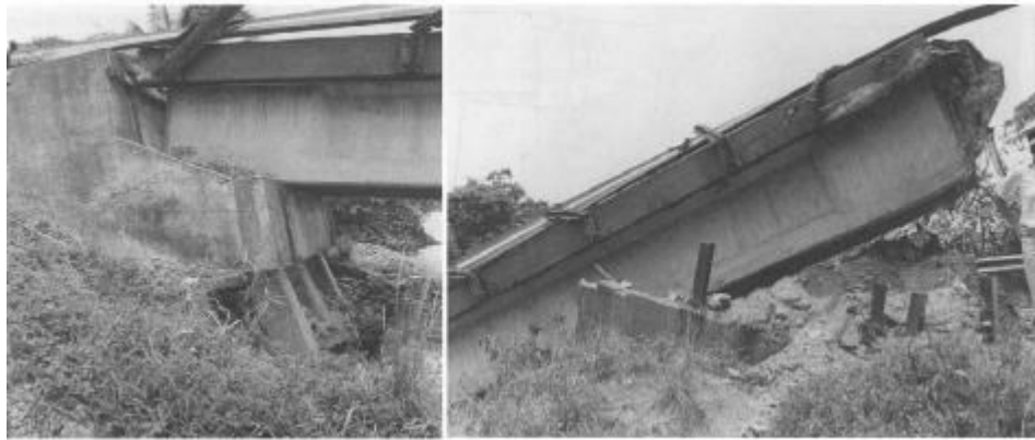
(a) (b) Figure 2-8 Two failure scenarios for the abutments: (a) due to slumping and rotation failure, Rio Banano bridge, 1990 Costa; (b) due to passive pressure, Rio Viscaya bridge, 1990 Costa
