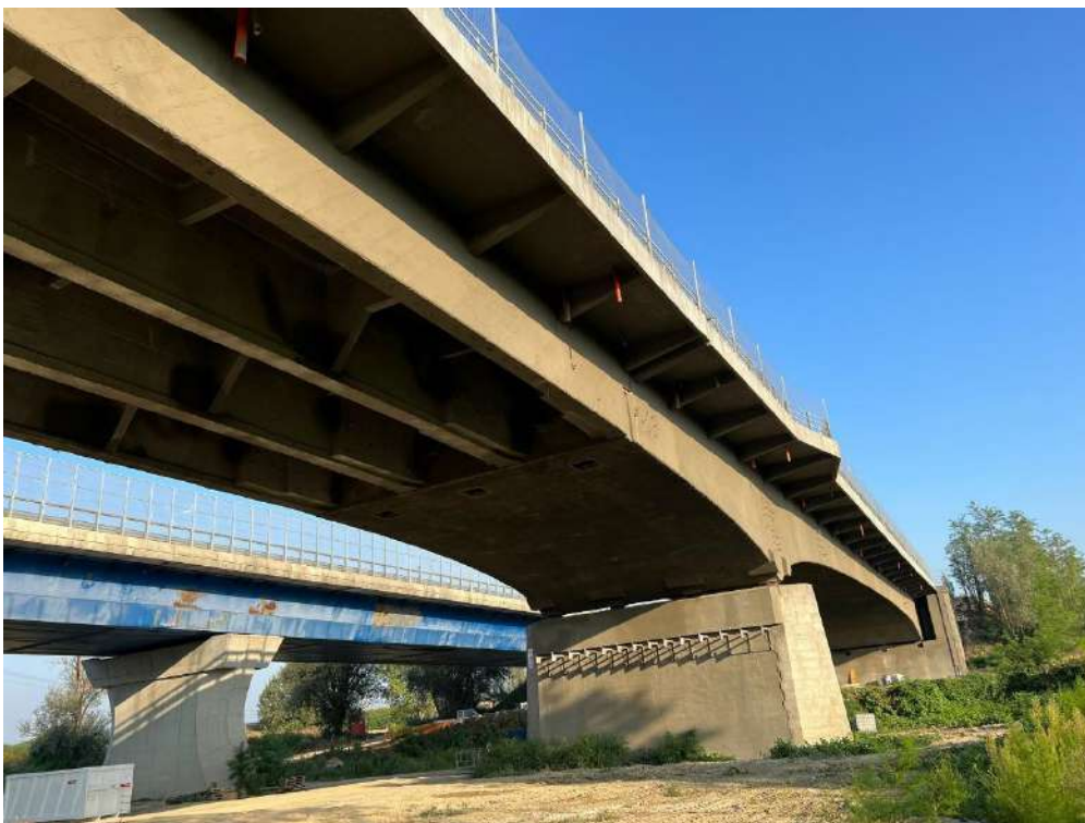
Figure 5.4: Side view of the underside of the Ponte Po – Careggiata Nord bridge structure.
